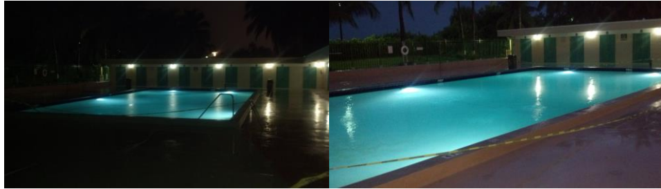
South swimming pool new illumination!
